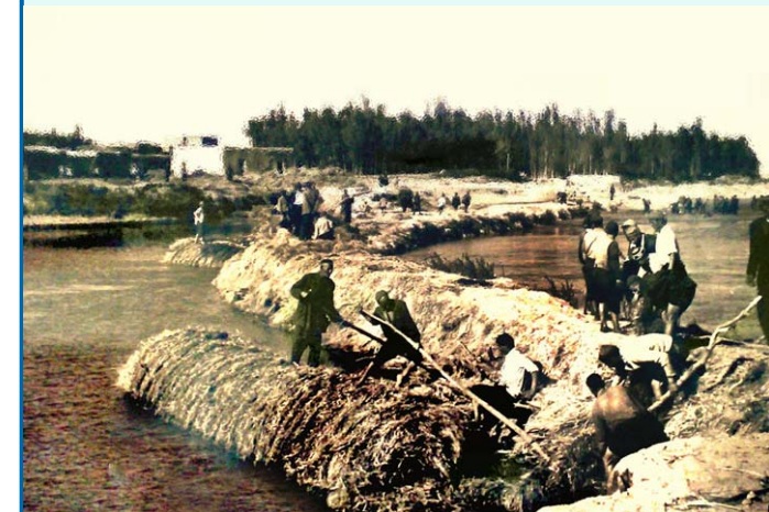
▲ Construction of A Diversion Dam on “Zarineh-Rud” River, Using Chaff as the Main Material; A Symbol of Creativity, Endeavor, and Team Work. North-Western of Iran, June 1965
